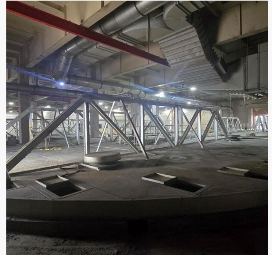
AlexRenew's gravity thickeners inside Building C
