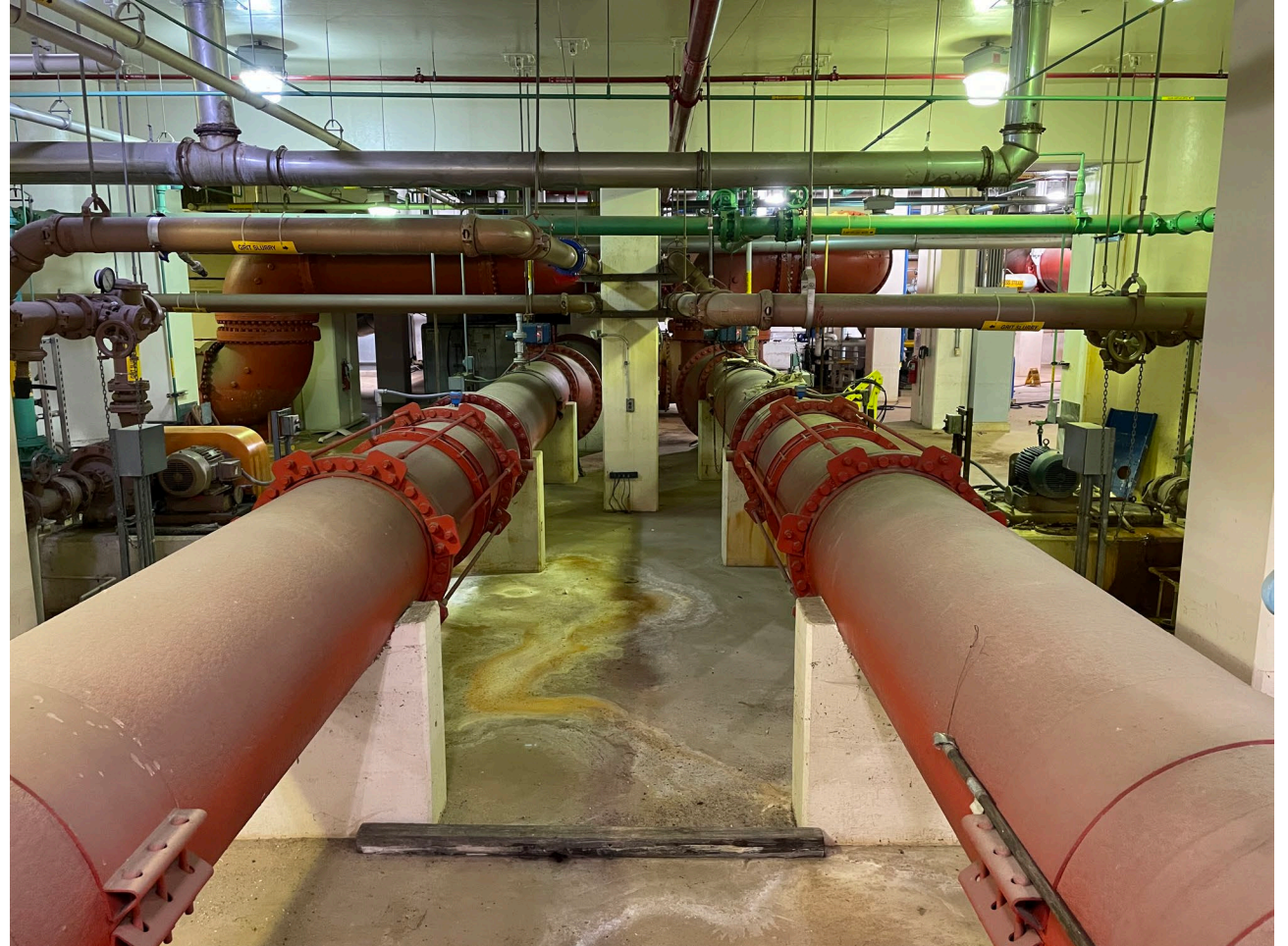
AlexRenew's Primary Influent Conduits in Building K
