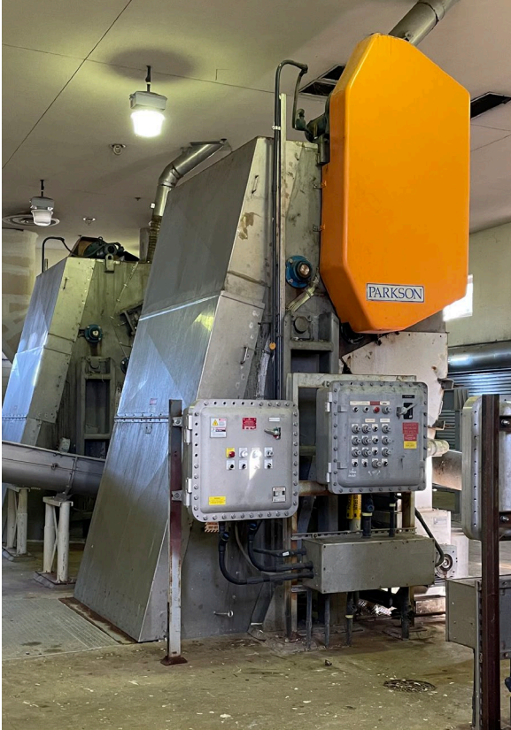
Upgrade two (2) fine screens
