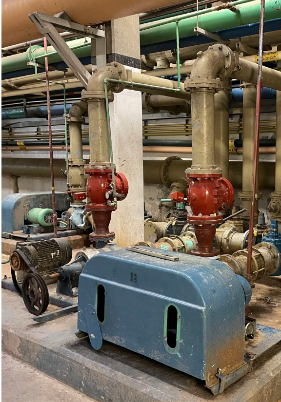
Replace twelve (12) primary sludge pumps
