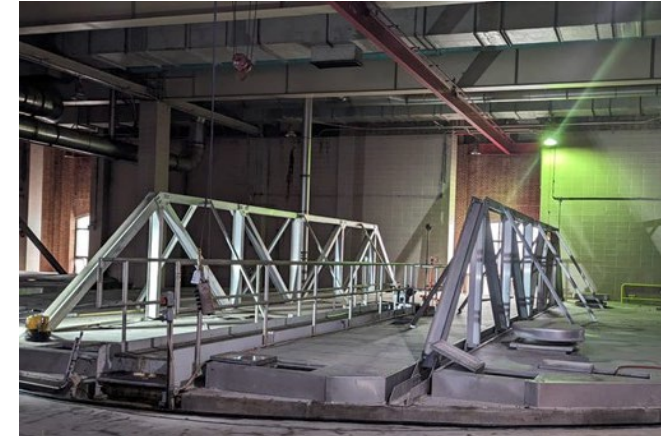
Existing gravity thickeners
