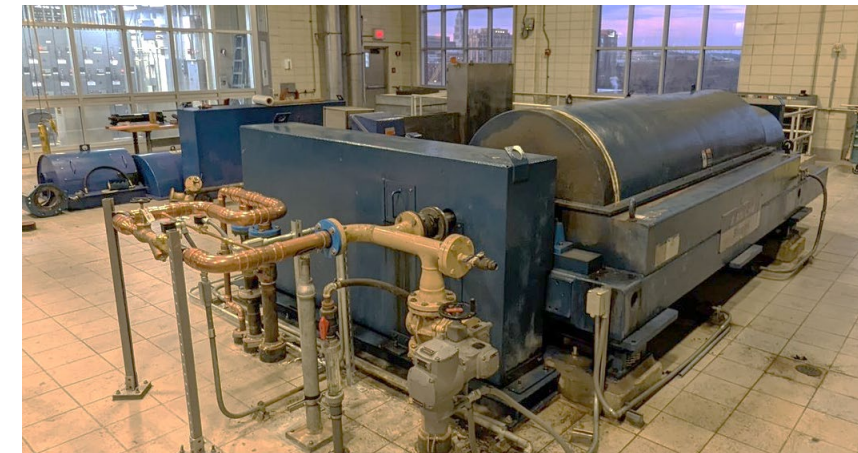
Existing dewatering centrifuges in Building L
