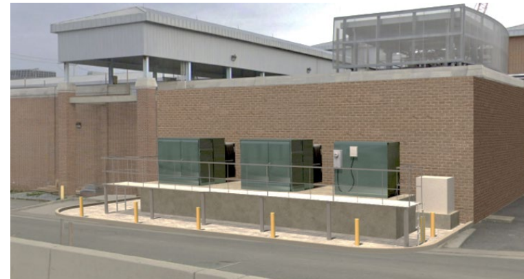
Conceptual location of new transformers, located south of Building 44
