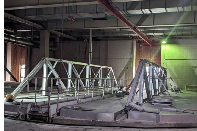
Existing Gravity Thickeners
